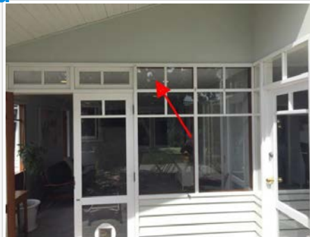
No head flashing
