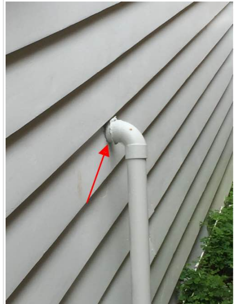
Penetration not sealed correctly.
