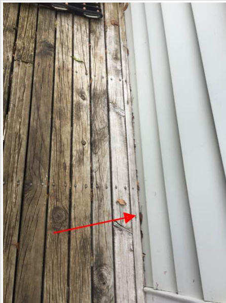
Decking in contact with cladding
