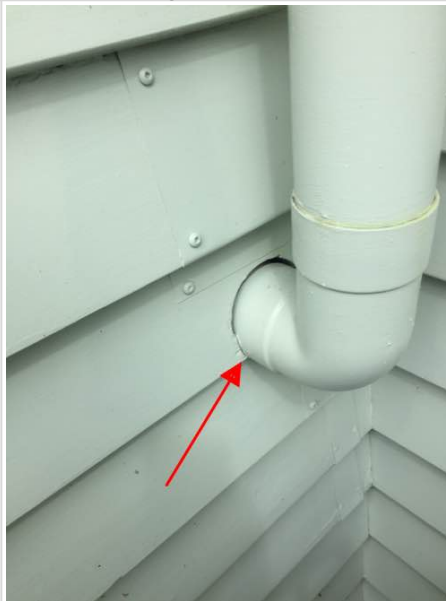
Penetration not sealed correctly
