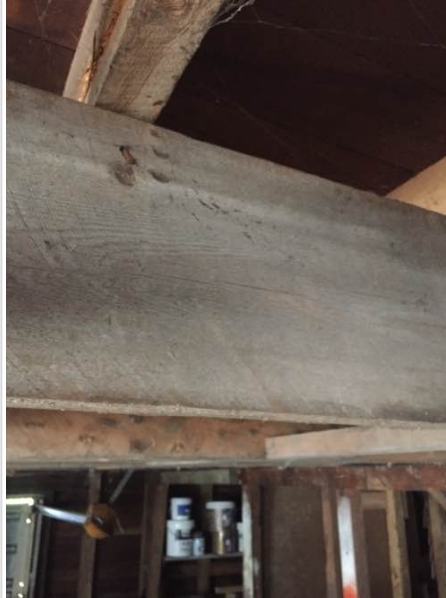
No evidence of borer or similar insect to timber at time of inspection
