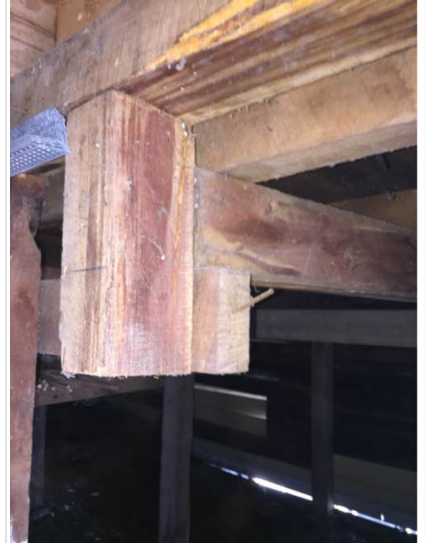
Appears a stud may have been cut to gain access under house. This area requires attention.
