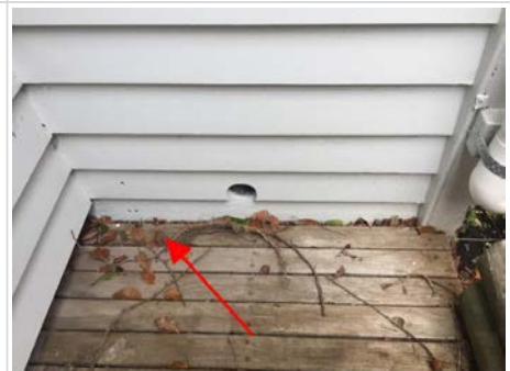
Decking in contact with cladding
