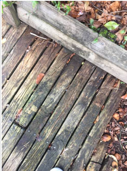
Decking to side of house is in poor condition
