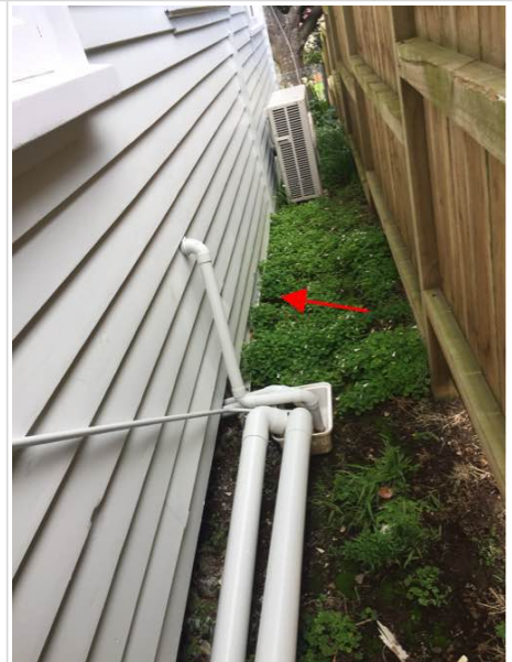
Ground and vegetation in contact with cladding. Maintenance required.
