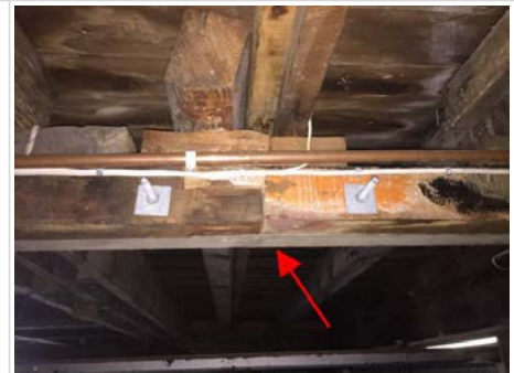
Join with no support under it. Requires attention.
