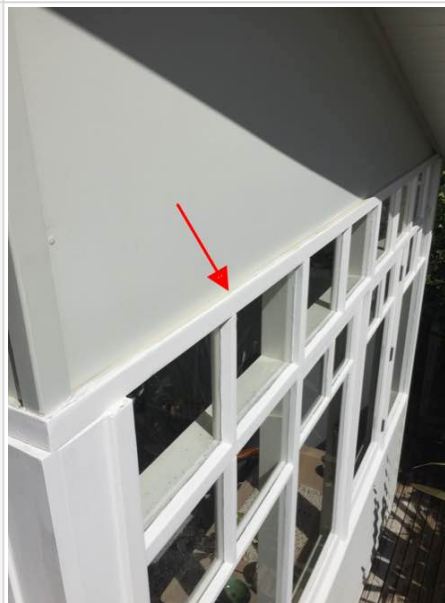
No head flashing
