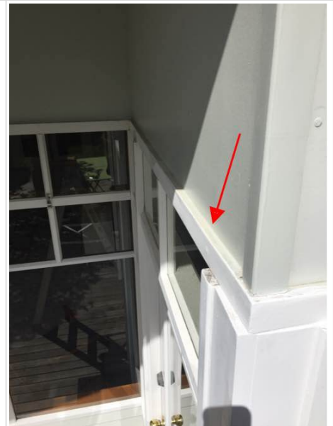
No head flashing
