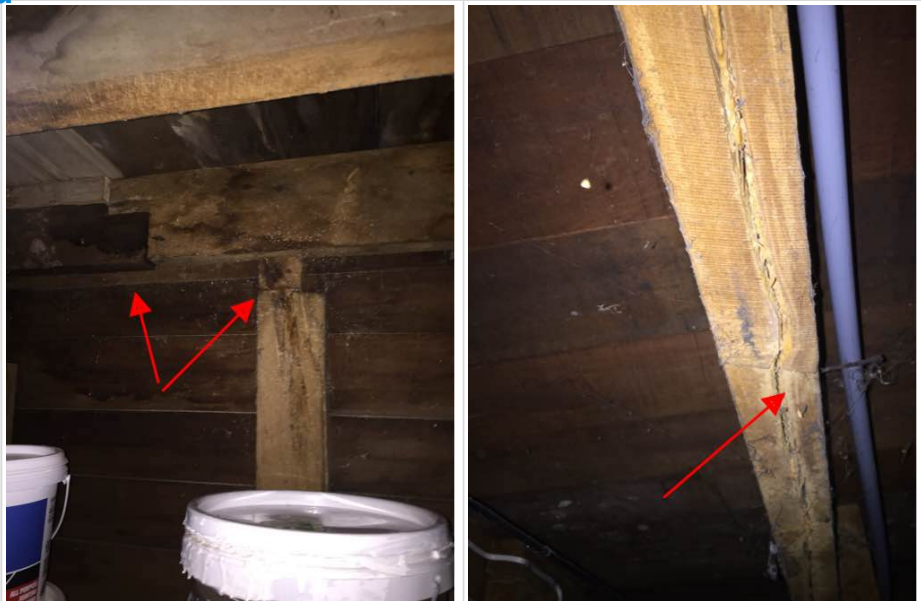
Packer under joist. No support under join. No mechanical fixings. requires attention.
